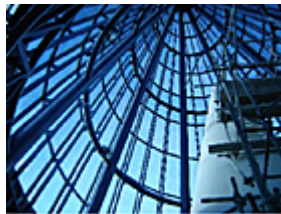
Khalifa Stadium in Doha, Qatar Using Lexan* Thermoclear* SunXP 25mm Sheet in Blue
